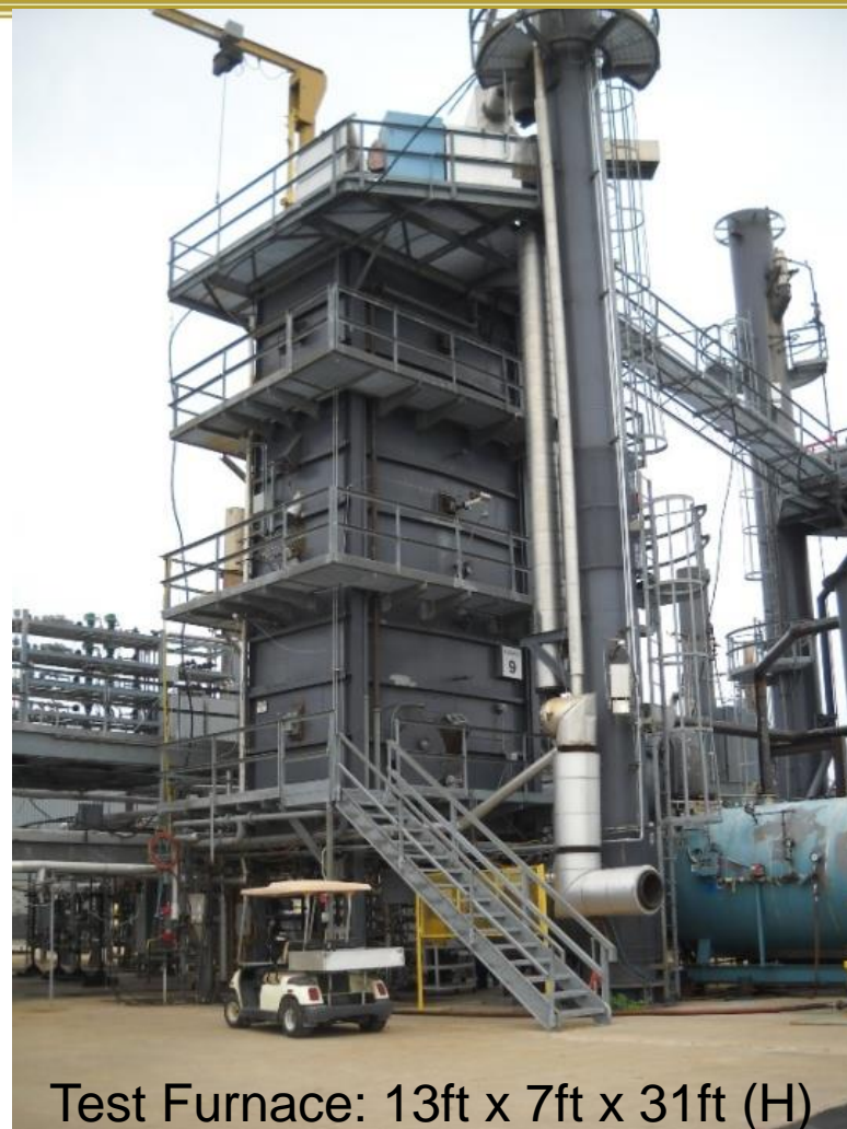
Furnace for burner tests (courtesy of John Zink Co.)
